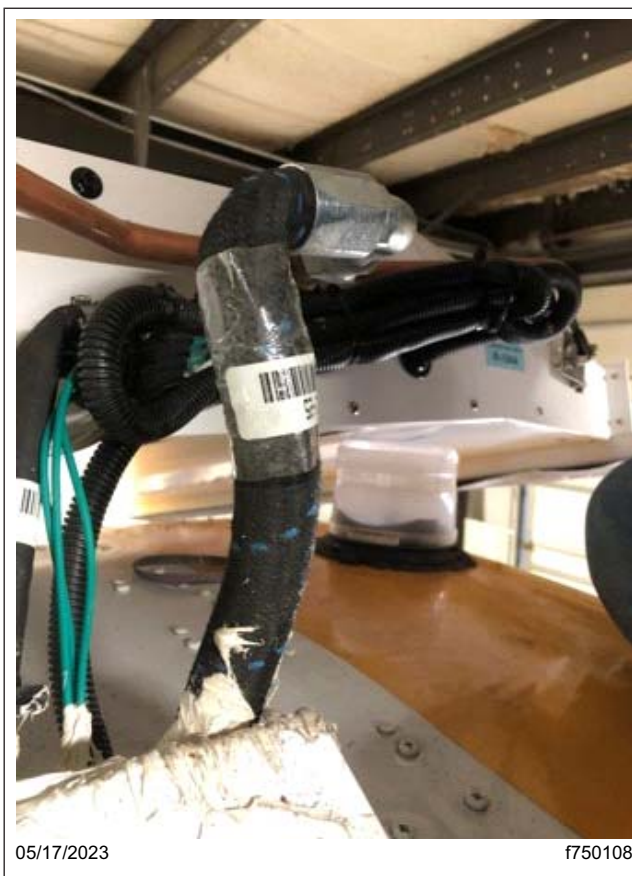
Fig. 7, Roof-Top A/C Plumbing
