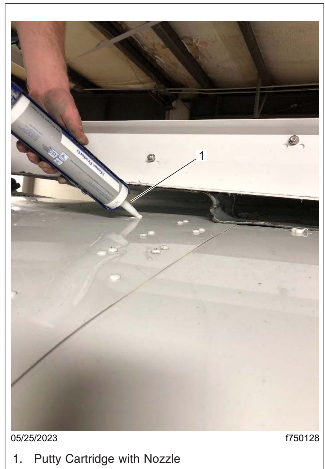
Fig. 6, Roof-Top A/C Sealed with Putty
