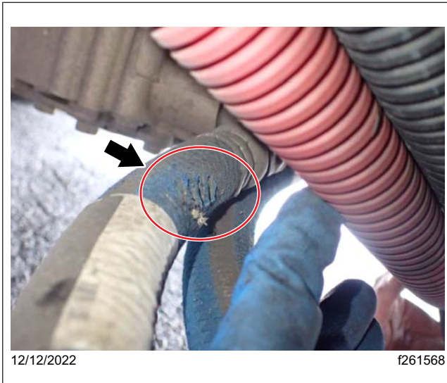
Fig. 1, Blemishes on the Power Cables and the Cooler Hoses
