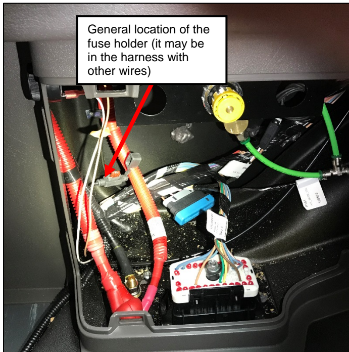
Figure 2: In-Line Fuse Holder Location
